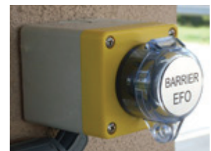
9. Exterior EFO Remote Control Panel
